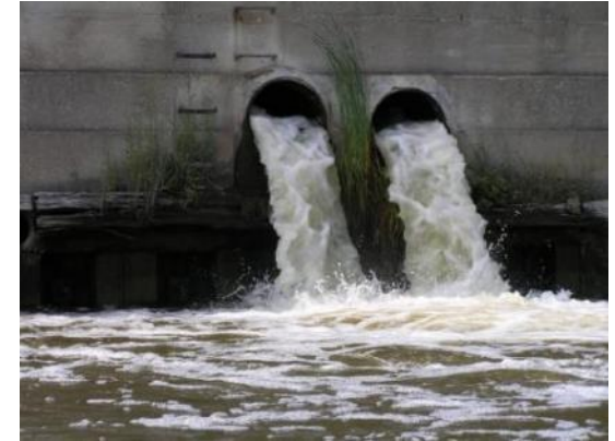
Combined Sewer Overflow Pollution
