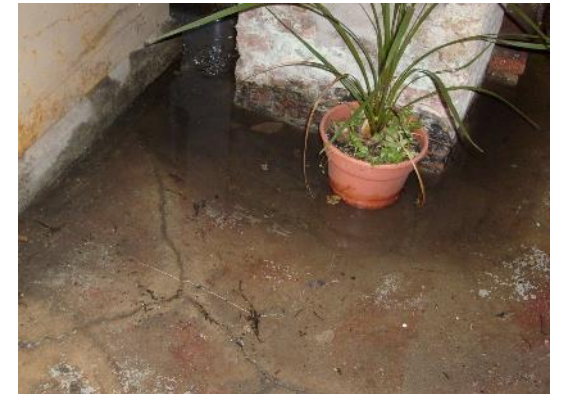
Seepage through basement walls/floors
